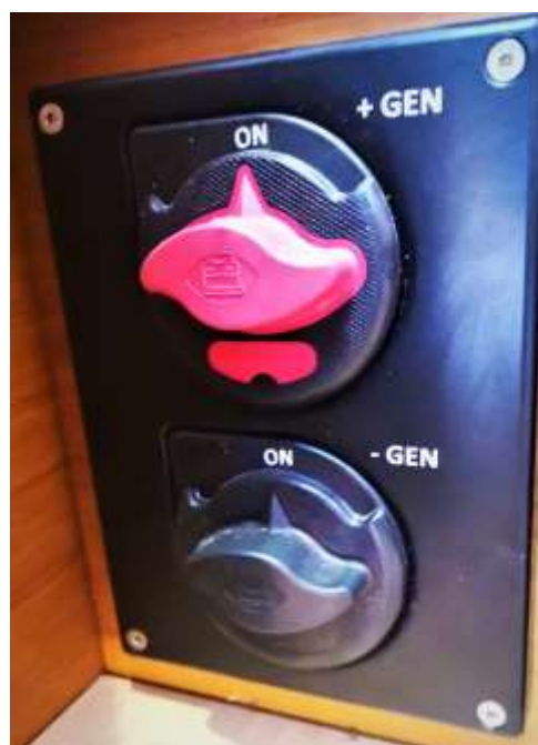
Generator Battery Switch
