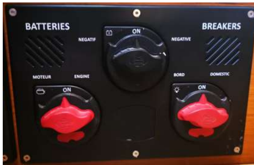
Domestic (Main) Battery Switch
